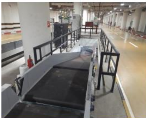
Baggage Breakup Area Conveyor Room
